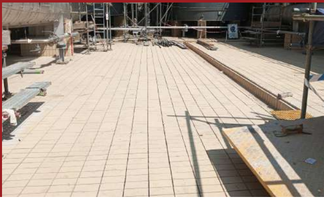
Acid Tiles - Msp Smelter
